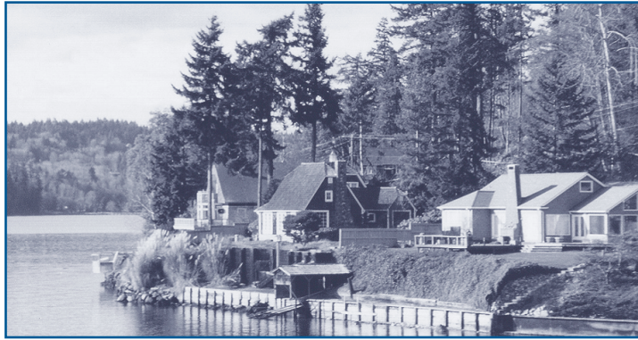
Bulkheads or riprap—such as those pictured above—that are used to harden shorelines can have the following effect on marine nearshore habitat:
