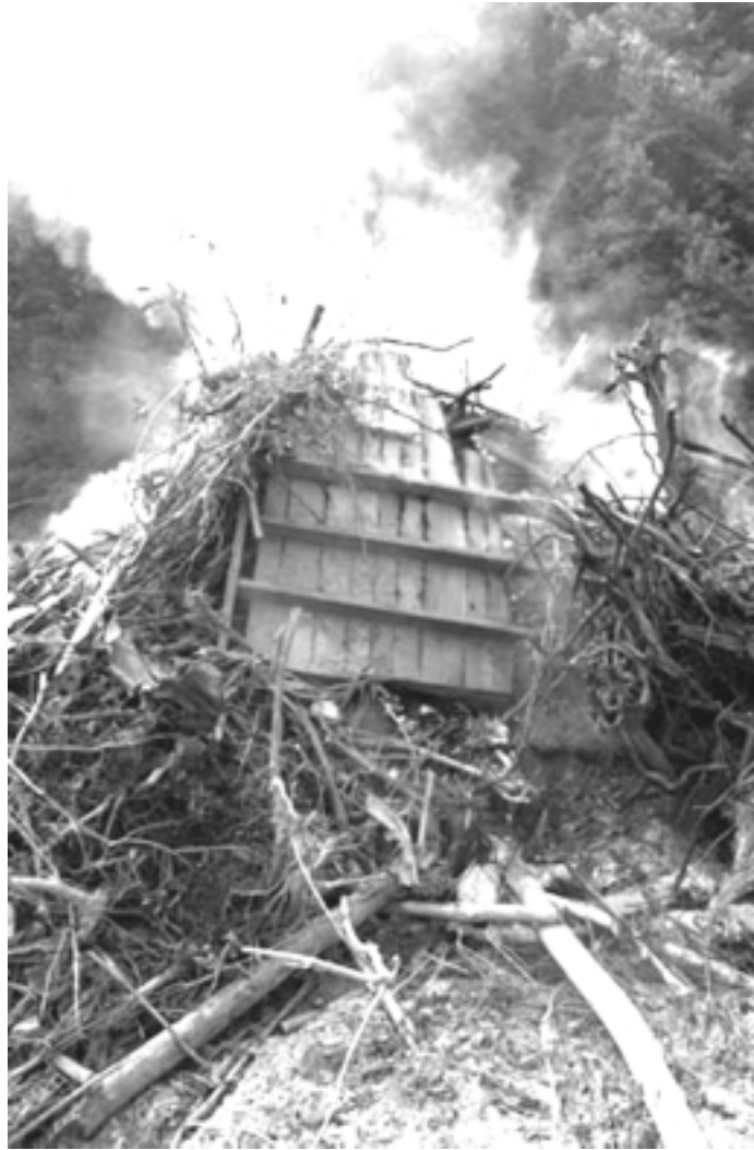
McGraw, WV, August 8, 2001— Road crews burn debris as a part of a clean up effort after recent flooding. Photo by Leif Skoogfors/FEMA News Photo
