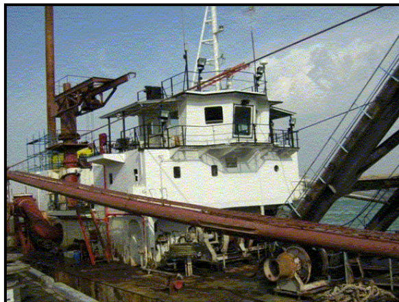
The Saif Sa'ad Dredger, rehabilitated by USAID, is performing maintenance dredging at Umm Qasr Seaport
