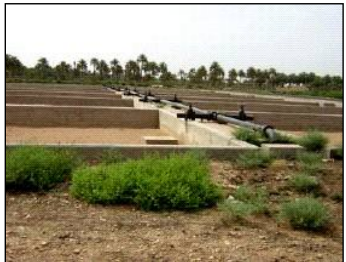
Sludge drying beds at Hillah wastewater treatment plant
