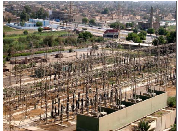
Baghdad's Doura power plant. USAID Photo.
