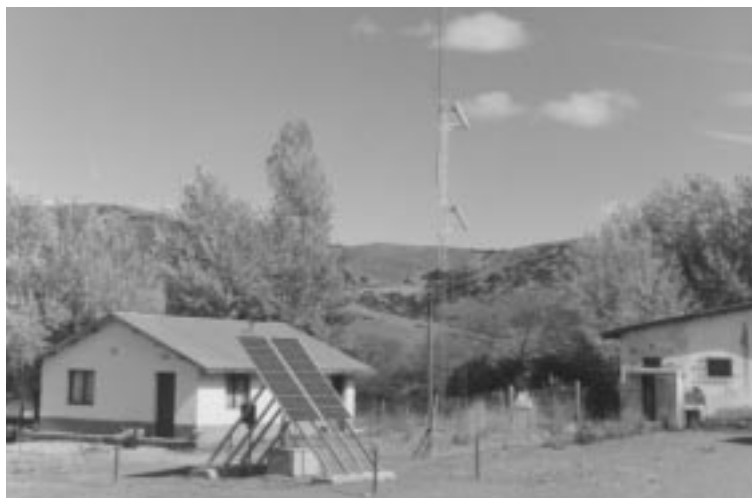
Figure 1.3. PV panels mounted on the ground and on a radio-transmitter tower.
