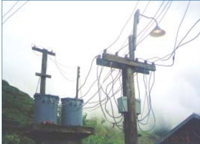
Transformers at the Tulgao-Dananao Micro-Hydro project, which provides power to 300 households
