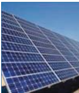
A PV panel
