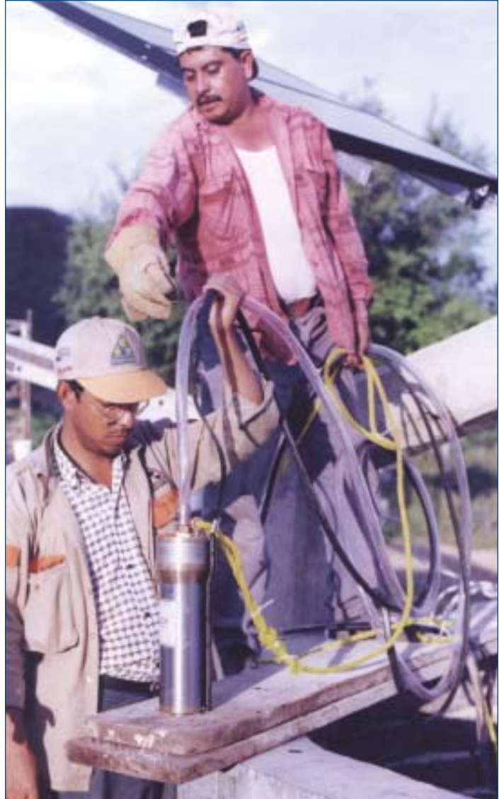
A PV powered water pump installation
