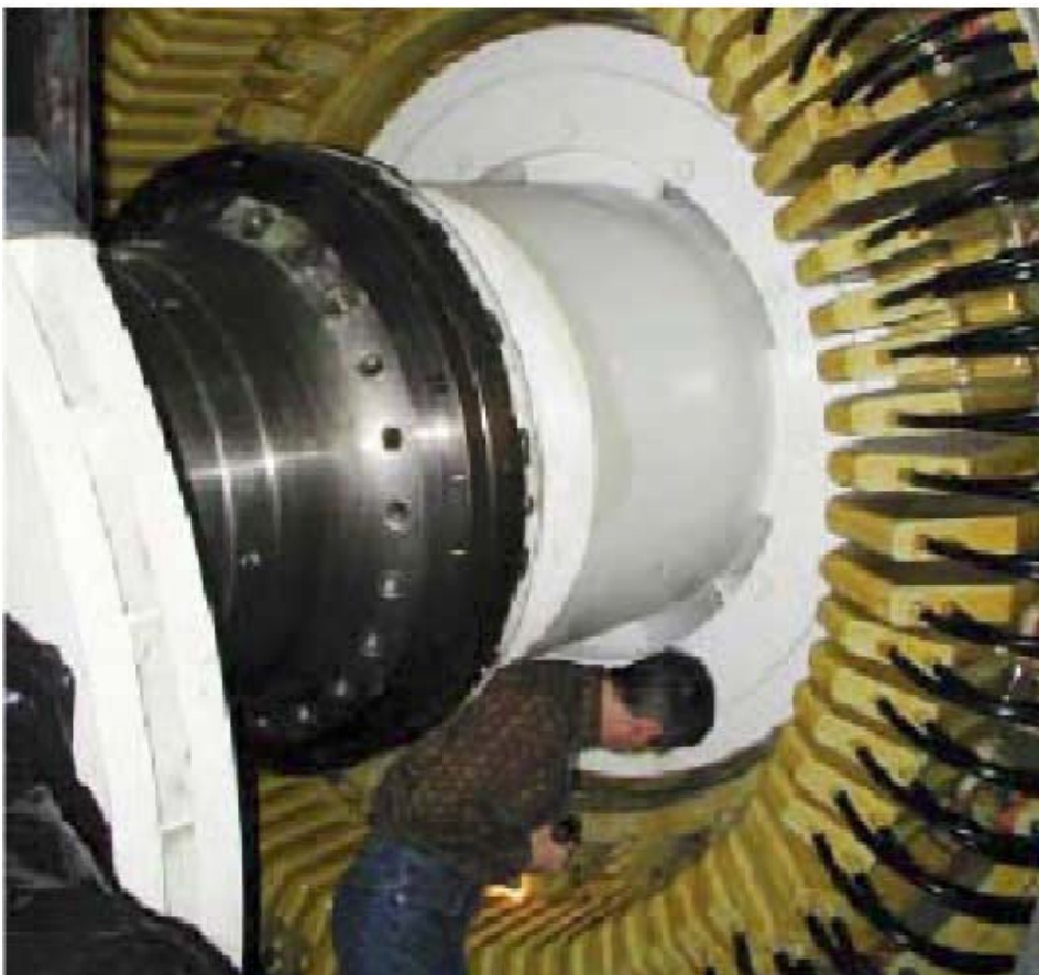
Inspecting the generator that is the largest among the magnet laboratory's magnetic-power sources.
