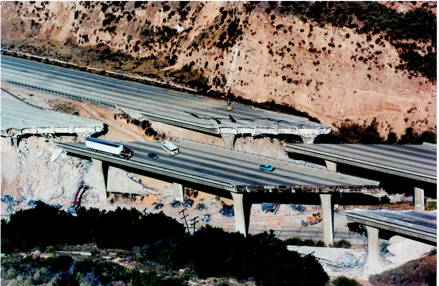
Figure 4. I-5 Damage at Gavin Canyon
