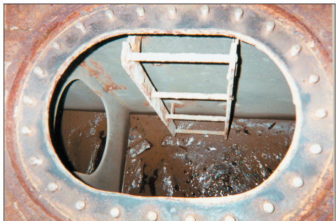
Looking into the entry hatch of a double-bottom ballast tank. Note accumulation of mud and water.
