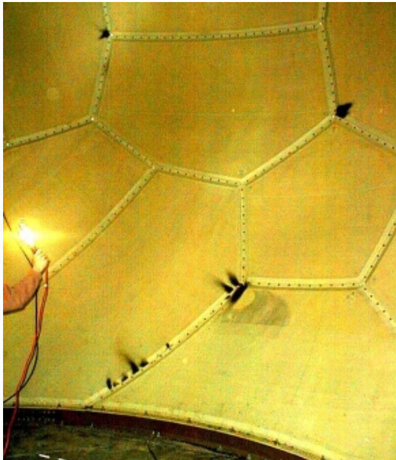
Figure 2. Burn marks on the inner surface of the radome of WSR-88D radar.
