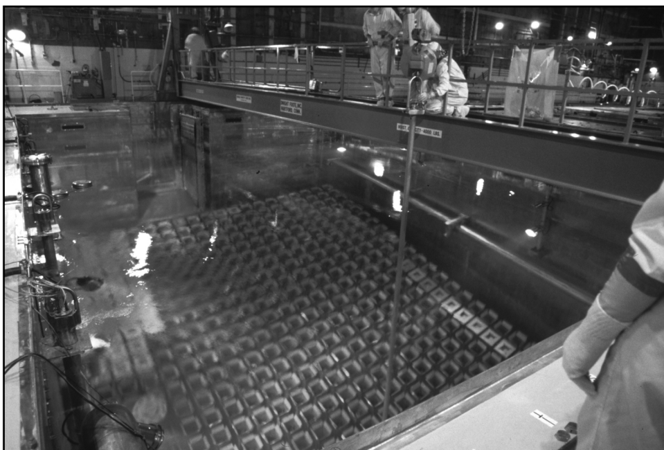
Figure 5: A Wet Storage Pool
