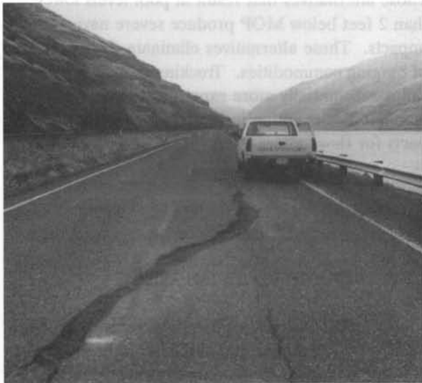
Figure 3-1. Typical Cracking in Whitman County Road 9000 after March 1992 Lower Granite Drawdown Test
