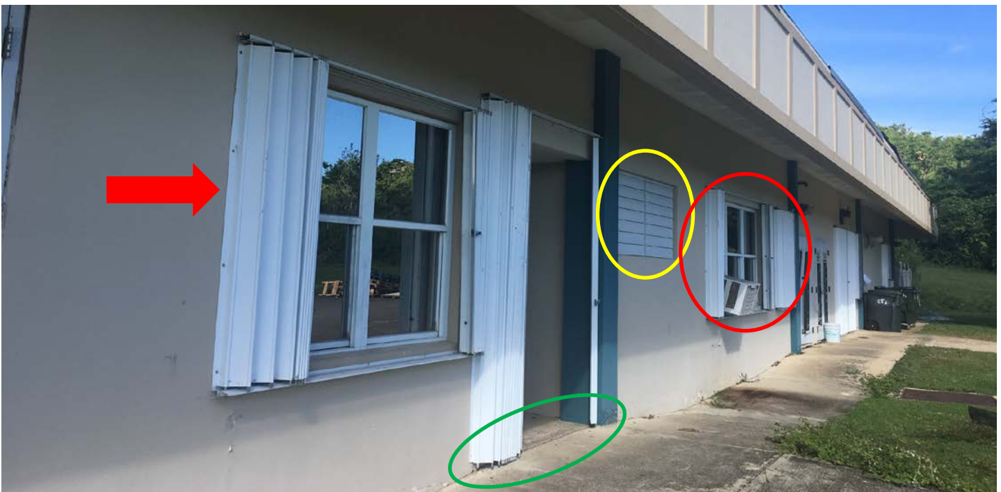
Figure 13. Installation issues that affected the performance of the impact-resistant systems include the lack of a bottom track (green oval), a window air conditioner preventing shutter deployment (red circle), and a metal jalousie opening with no impact-resistant system (yellow circle).
