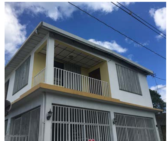
Figure 10. A two-story residence with windows and gill doors (upper porch) protected with metal panel shutters.
