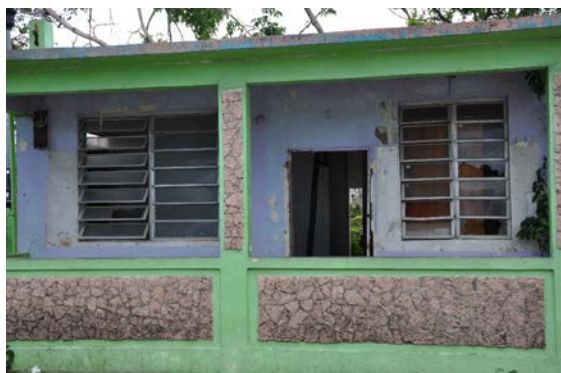
Figure 2. Residence where unprotected glazing louvers were broken by wind-borne debris on the left and right sides of the entry door.
