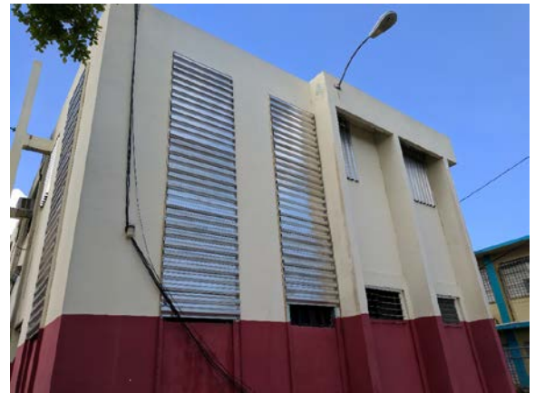
Figure 12. A fire station with metal panel shutter system deployed provided adequate protection for the facility.
