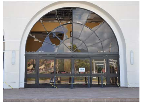
Figure 9. Glazing damage at the main entrance to a community building/convention center.
