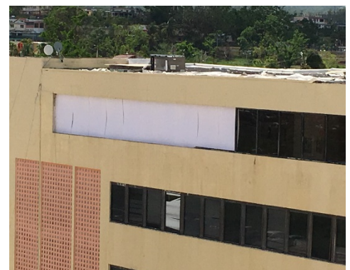
Figure 8. An entire bay of windows is missing from the upper floor of this hospital in Bayamon due to a lack of adequate fasteners.
