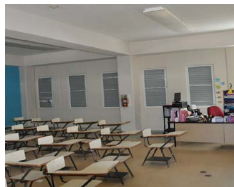
Figure 4. High school in a coastal community with metal jalousie openings. Screens were installed behind the jalousie openings.
