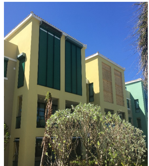
Figure 1. Residential windows protected (left) and unprotected (right). The unprotected windows were damaged and are temporarily covered with plywood.
