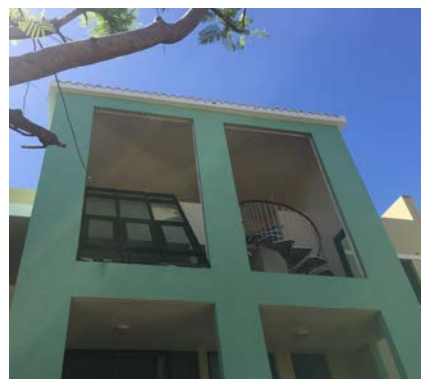
Figure 7. Two-story window assemblies (fixed and operable) failed at the frame-to-wall connection due to lack of proper fasteners.
