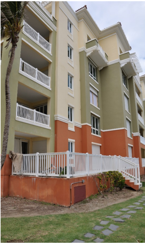
Figure 5. Numerous operable casement and awning windows were damaged due to wind pressures and wind-borne debris at this waterfront building.
