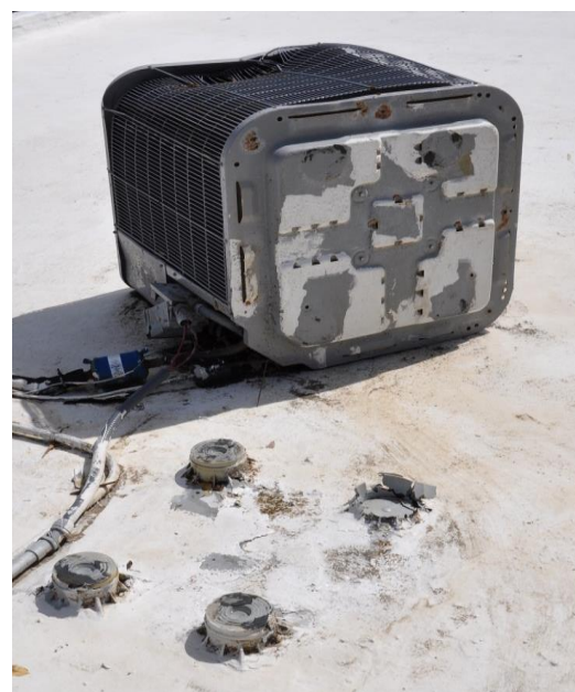
Figure 9. This condenser was blown off the plastic pedestals to which it was attached. One of the pedestals was broken (red arrow).
