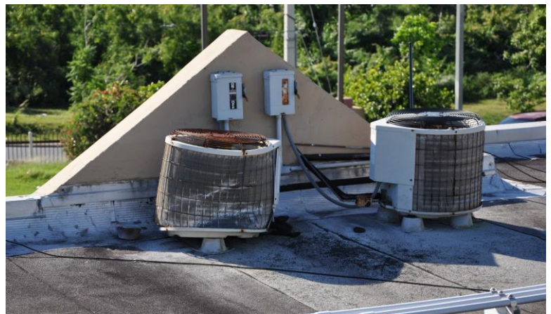
Figure 3. Rooftop AC condenser damaged by impact.
