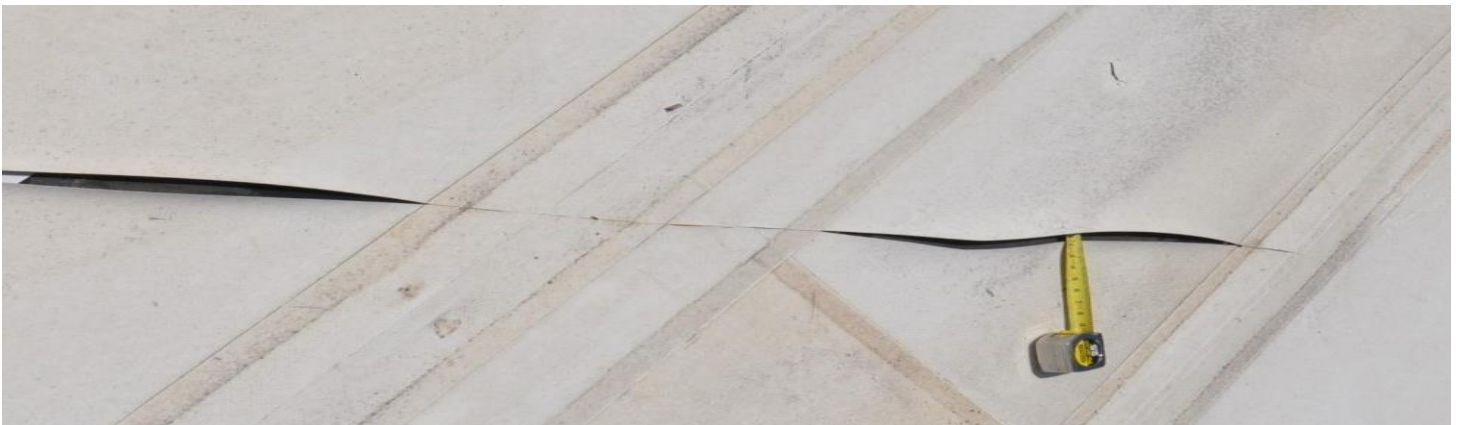
Figure 6. A tear several feet long in a roof membrane. Hurricanes Irma and Maria, U.S. Virgin Islands.
