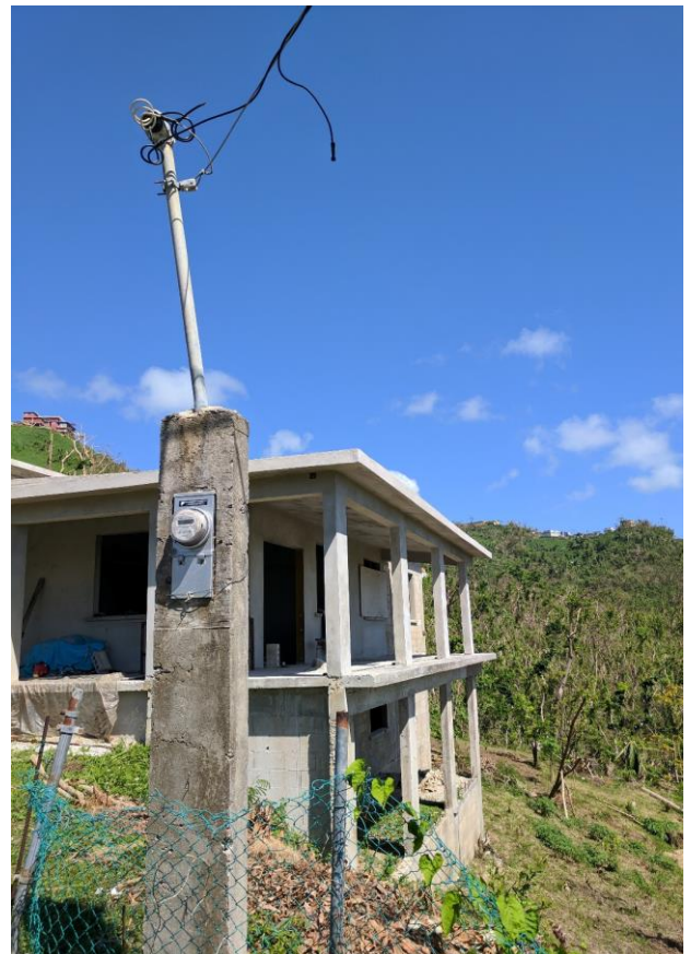
Figure 15. Power delivery pylon for the electrical service mast for a house under construction. The FEMA MAT frequently observed this installation method in Puerto Rico.
