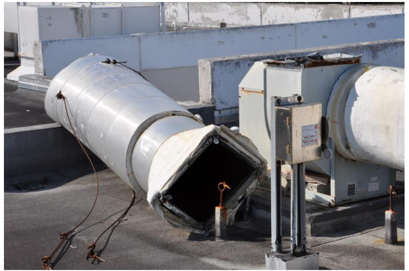
Figure 11. Toppled exhaust stack at a high school in Loíza.
