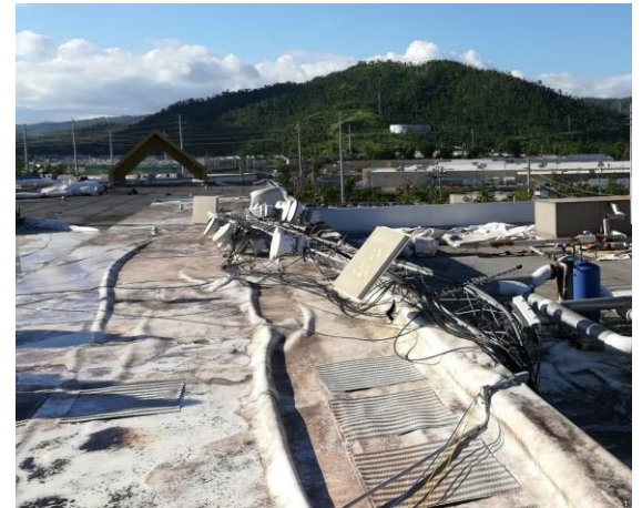
Figure 17. Collapsed roof-mounted antennae which had been inadequately secured to the roof using CMUS as ballast.
