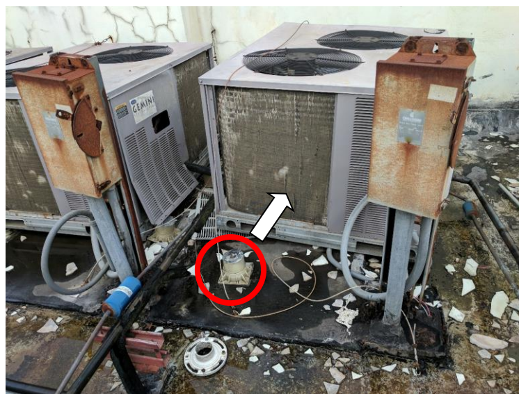
Figure 1. HVAC unit moved by wind. The unit was inadequately attached to the plastic pedestal (red circle).
