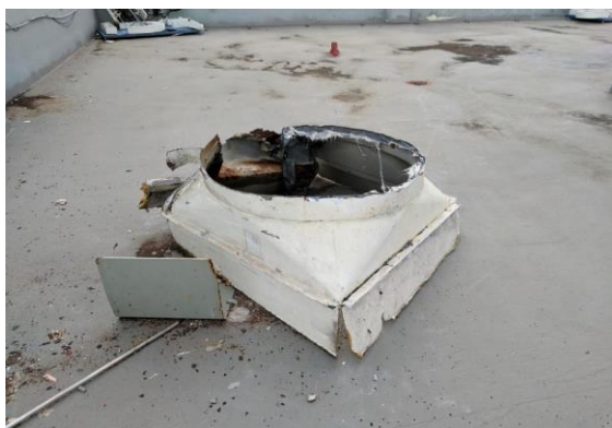
Figure 7. Blown off fan cowl resting on the roof membrane at a hospital.
