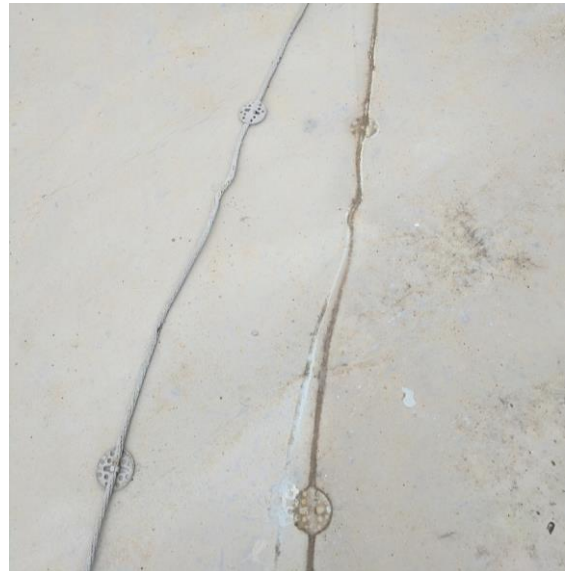
Figure 18. Detached LPS conductor that had been inadequately attached using adhesive.
