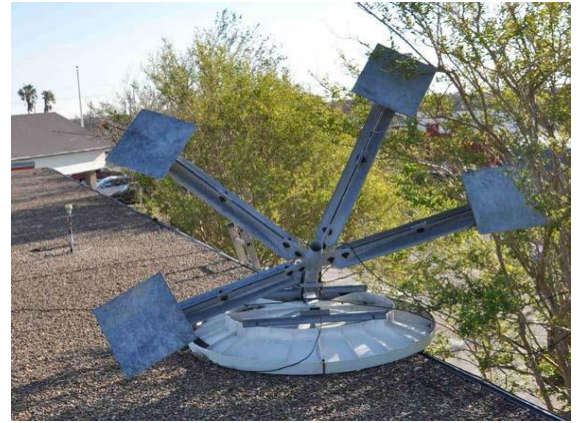
Figure 16. The satellite dish at this hospital was nearly blown off the roof. Hurricane Harvey, Texas.
