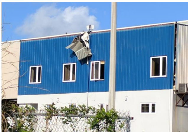
Figure 2. HVAC unit blown off a roof.
