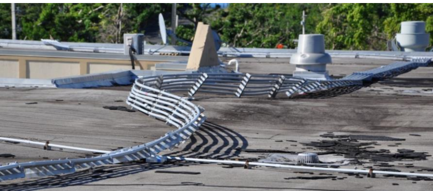
Figure 12. This conduit carried conductors from a rooftop solar array on the roof of a hospital in Vieques. It was inadequately secured to the roof and failed.
