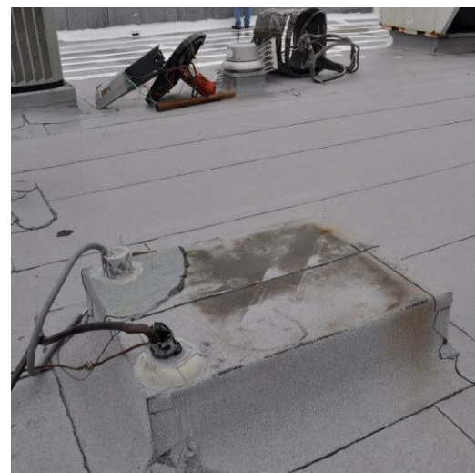
Figure 8. The condenser at this hotel simply rested on the curb. Hurricanes Irma and Maria, U.S. Virgin Islands.
