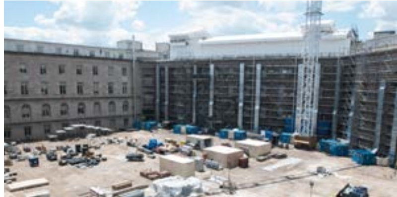
Exterior construction of the Cannon House Office Building. Photo by Kristie Boyd.
