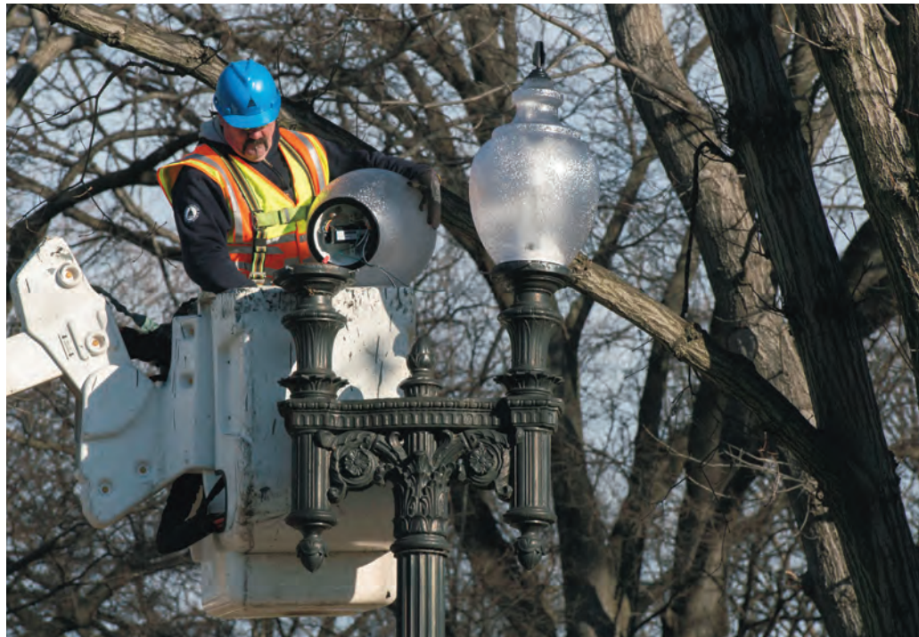
Berry Russom, High-Voltage Electrician Leader, works on a streetlight. Switching to high-efficiency lamps across the campus is one way the AOC has reduced energy consumption by 30 percent within 10 years. Photo by Susanne Bledsoe
