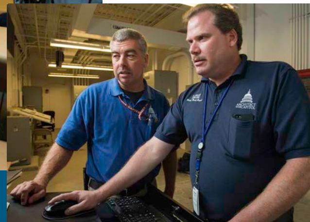
Scott Bieber and Andy Selby review the building automation system at Ft. Meade.
