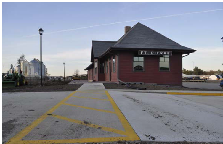
Half-a-million dollars are being spent to refurbish a decommissioned train depot in South Dakota which was being used a farm building.
