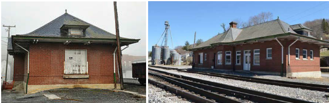
More than $300,000 is being spent to renovate this train station that has not served passengers in nearly 60 years in a Virginia town with fewer than 5,000 residents.
