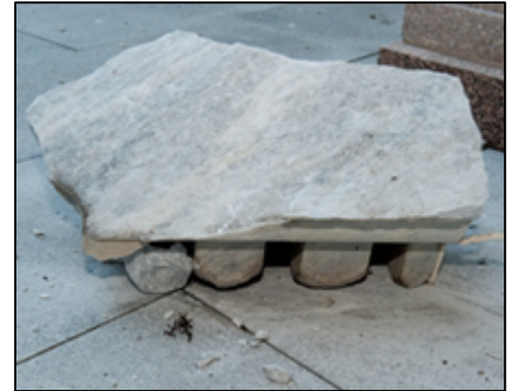
A large piece of stone that fell from the Capitol Building.
