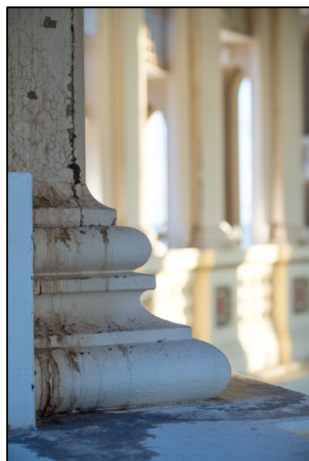
Water infiltration into the Rotunda has caused damage to cast iron columns and threatens historic artwork.
