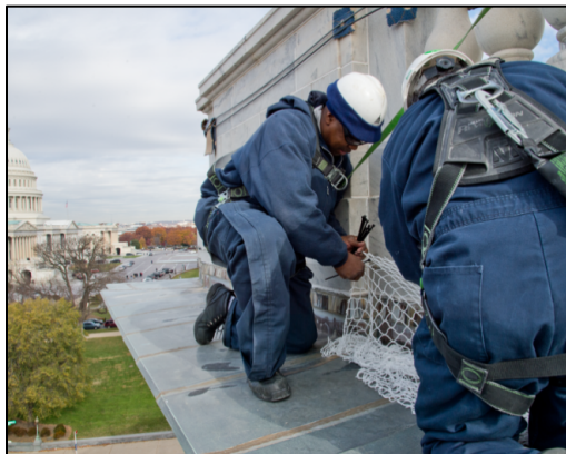
AOC employees install netting on the Cannon Building to prevent additional stone from falling.
