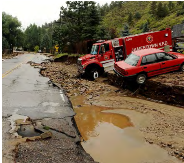
Road washed away by extreme flood in Jamestown, Colorado
