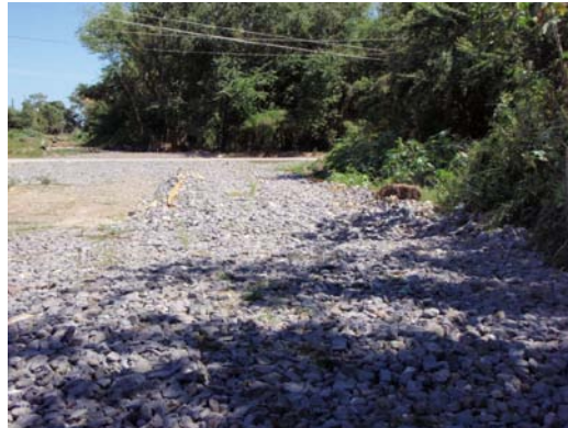
Tire washing station
