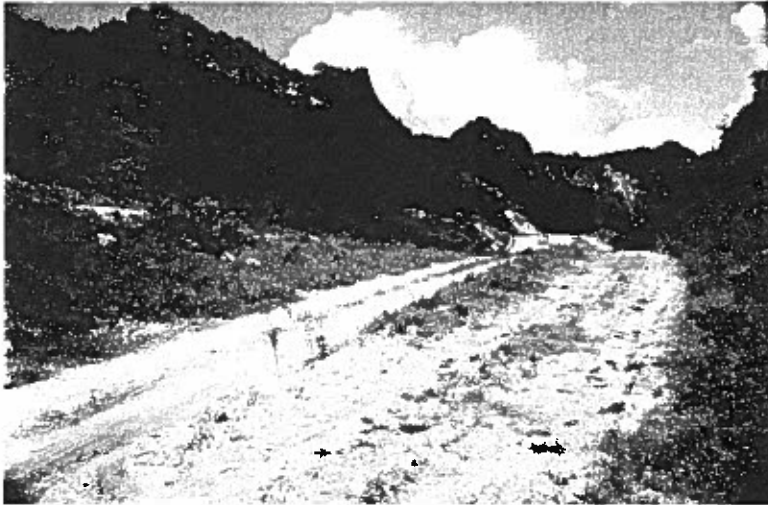
Figure 2. The photograph shows PR-10 under construction. On the background Lares limestone cliffs are shown..
