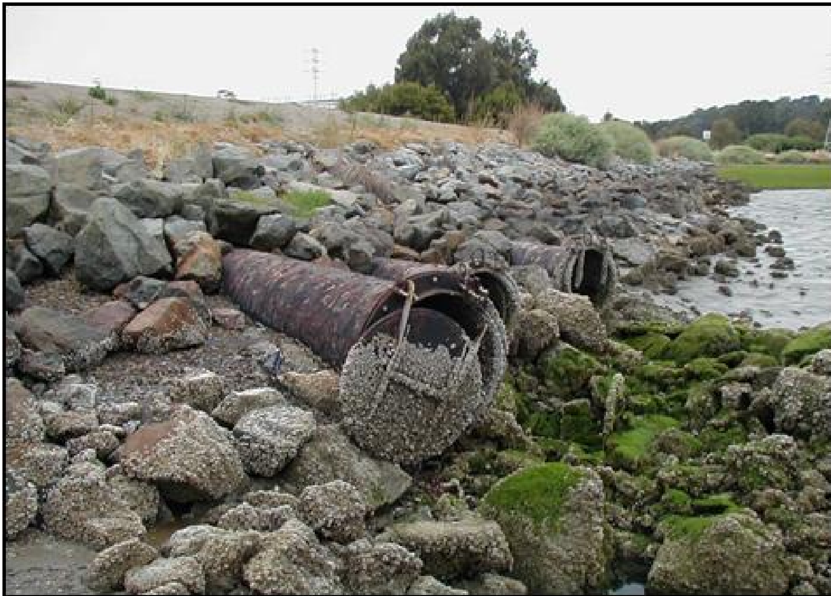
Poplar Pump Station existing outfall pipes to Bay
