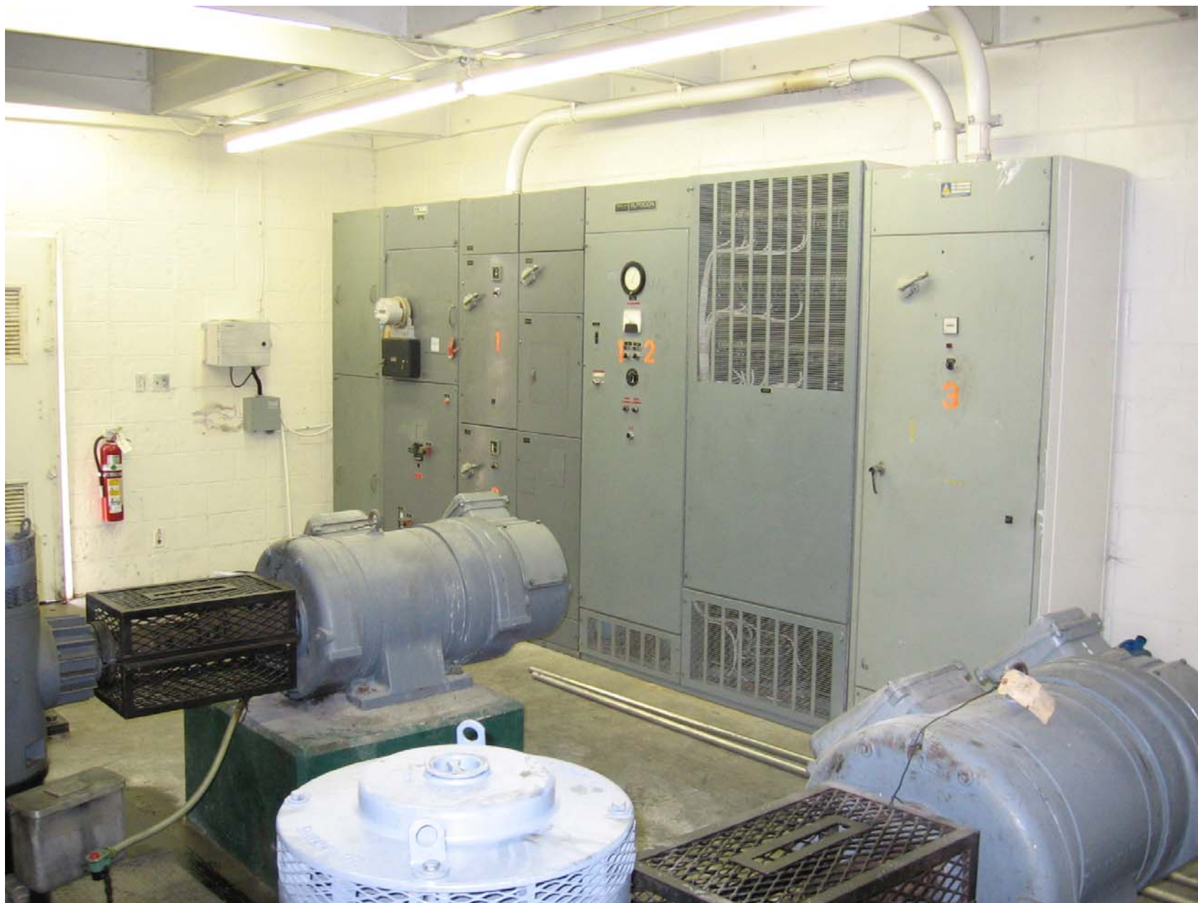
Poplar Pump Station Interior
