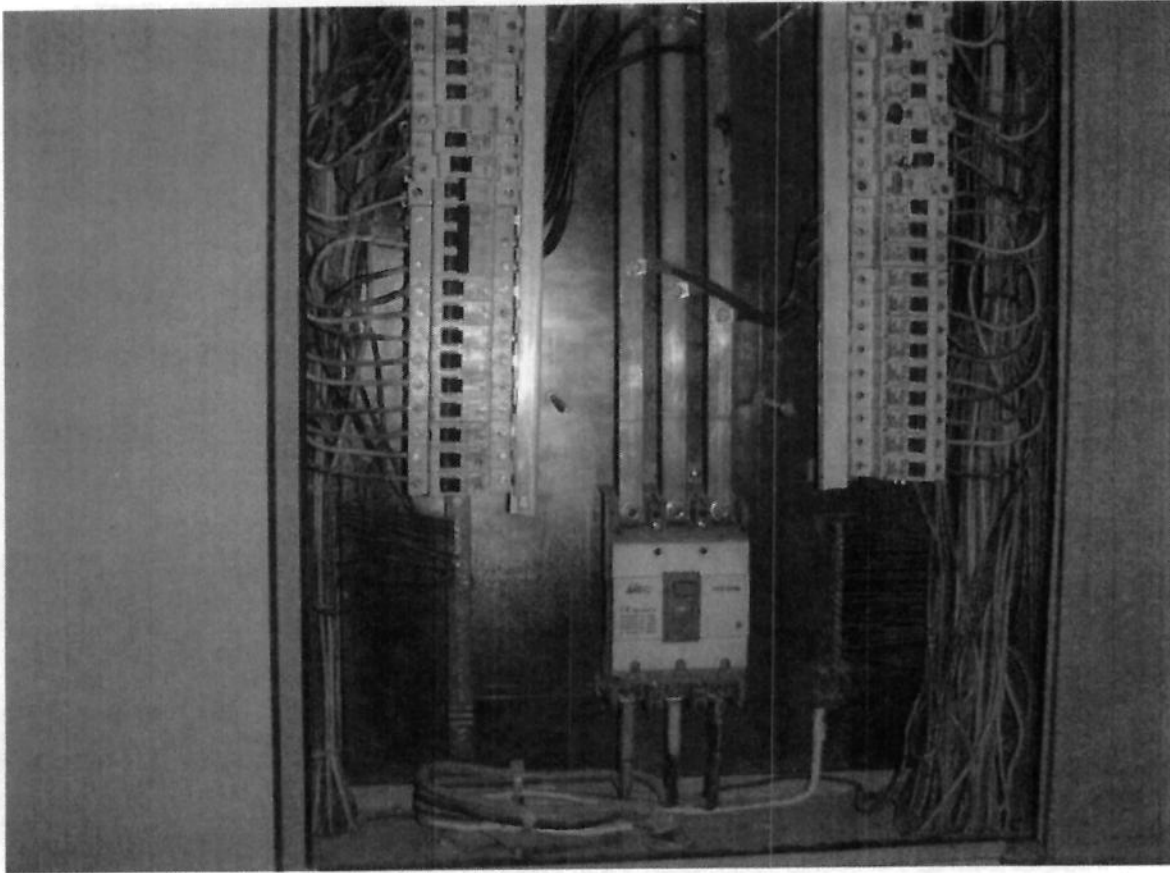
Figure 3 BLDG 11. Four wires coming in, no bonding of neutral to ground and no ground electrode conductor.
