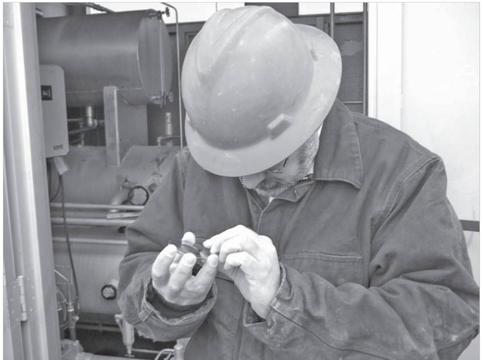
Figure 8: BLM Petroleum Engineer Technician Inspecting an Orifice Plate
