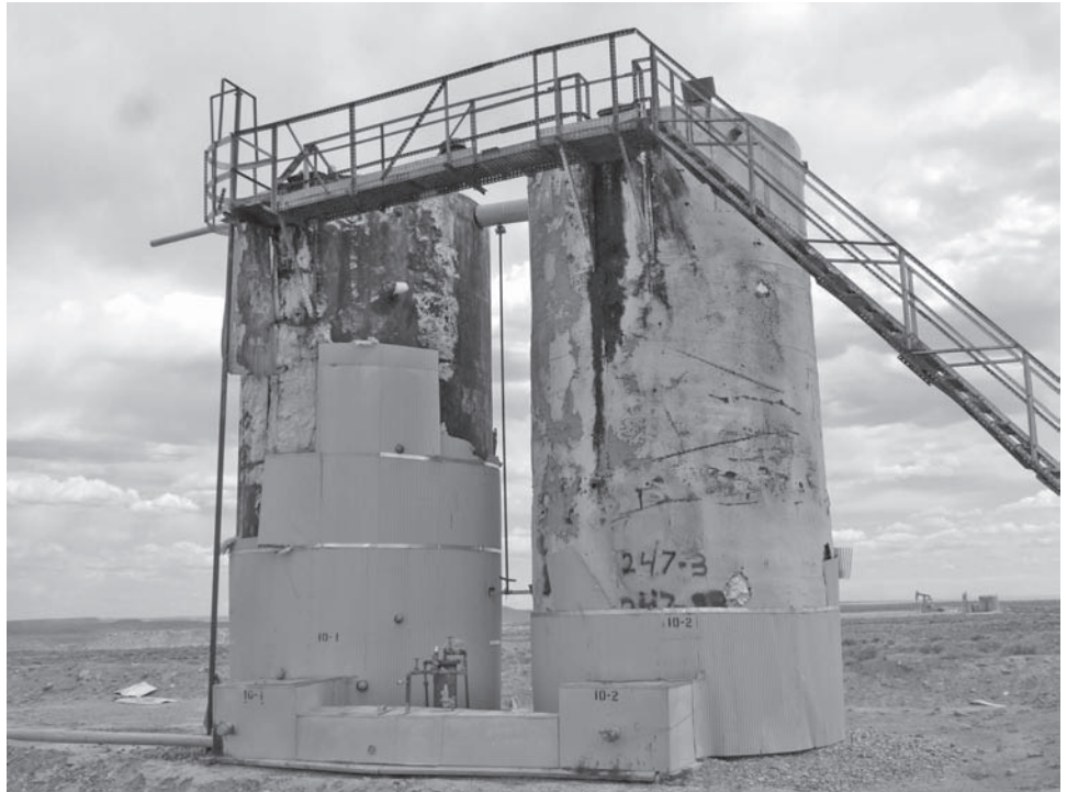
Figure 7: Oil Storage Tanks that Had Not Been Inspected for Several Years
