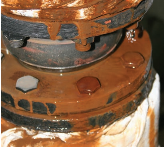
Evidence of water leakage from hot-water line.
