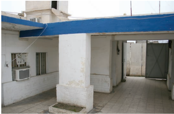
Improperly strung electrical wiring.
