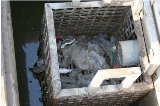
The adequacy of the piping system was demonstrated by the fact that medical waste materials managed to make their way through the piping system.
