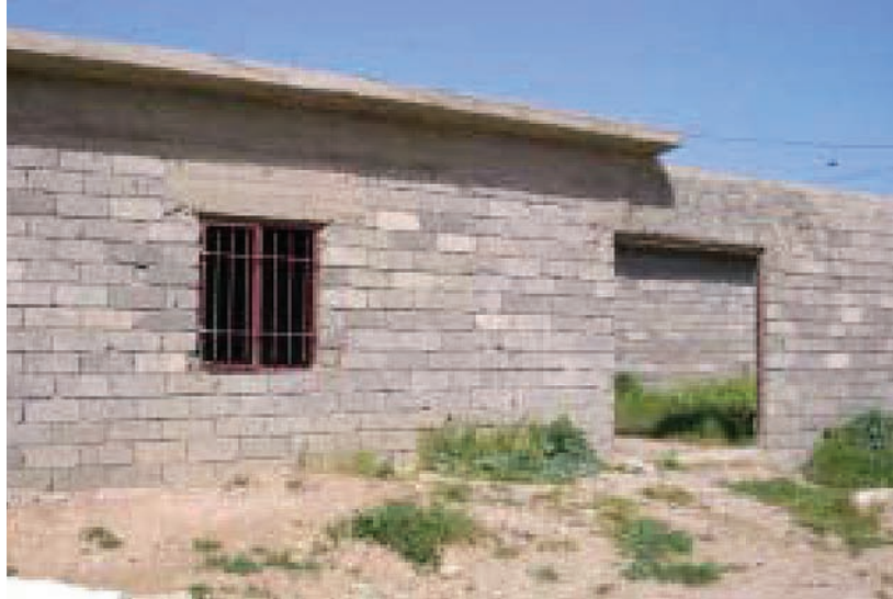
Renovation work included installing a floor, detention cell, and steel bars over windows.
