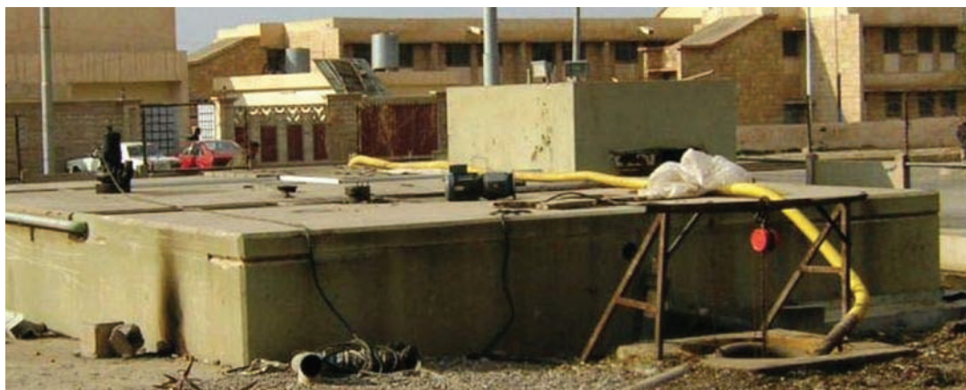
Before renovation, the septic tank was bypassed and hospital sewage was pumped from the cesspool to the municipal system. (USACE, January 4, 2005)
