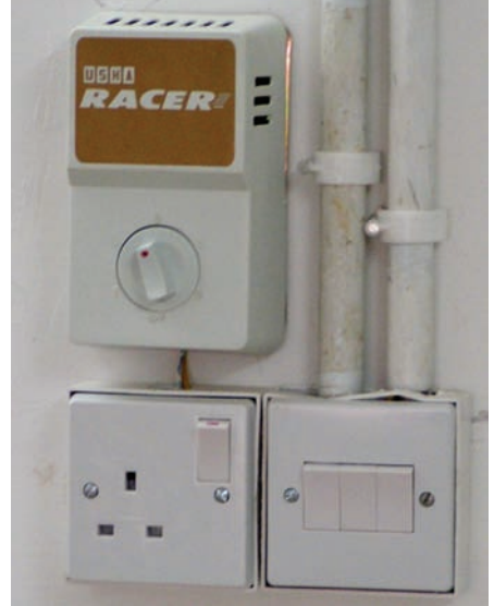
Wiring and components securely fastened to walls.
