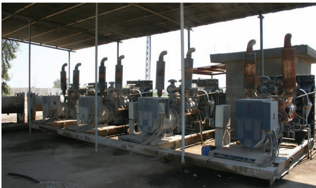
Four generators installed, but not operational during site visits.
