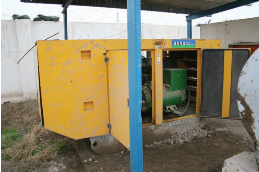
Abandoned generator with no fuel line, low oil levels, broken working-switch gears and controls.
