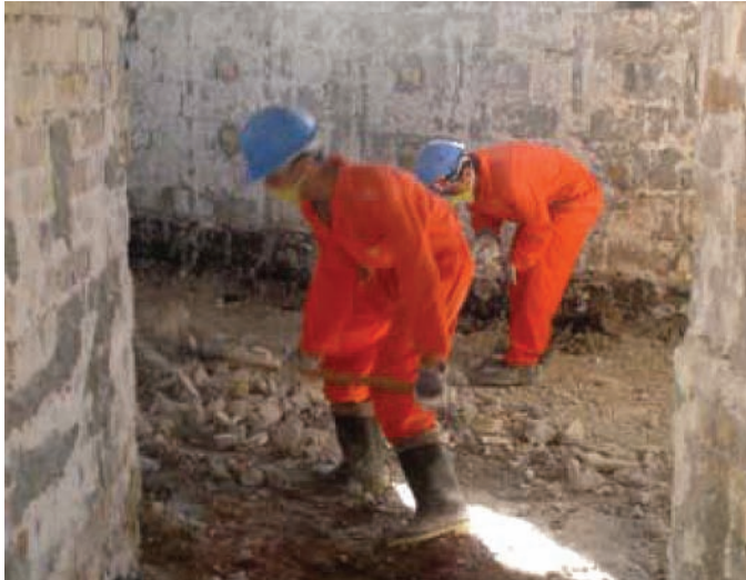
Waste from plugged external toilets was removed from the floor by workers prior to renovation. (USACE photo, June 18, 2006)
