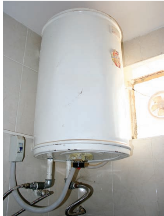
Water heater installation with metal piping and fittings, and a breaker/switch.
