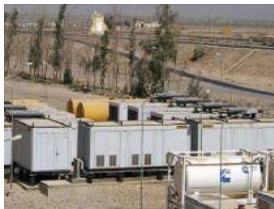
Seven Caterpillar generators. (Photo provided by USAID)
