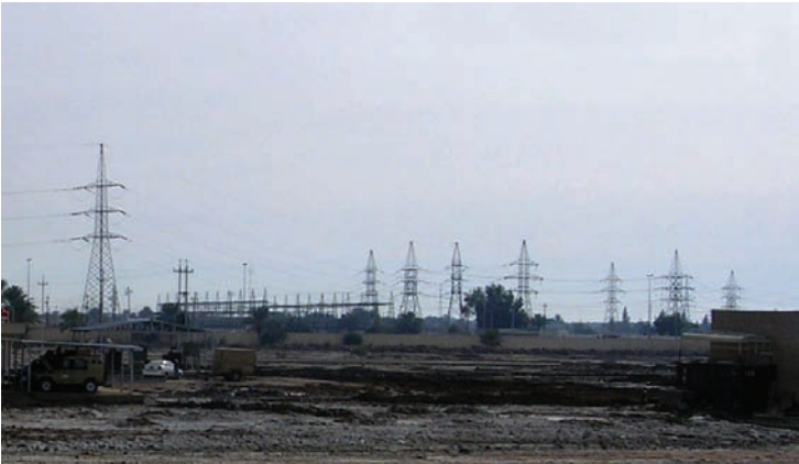
Protecting the linear infrastructure in the electricity sector remains a challenge across Iraq.
