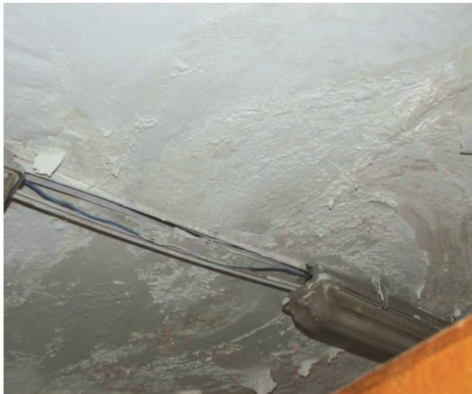
Water damage to the ceiling.
