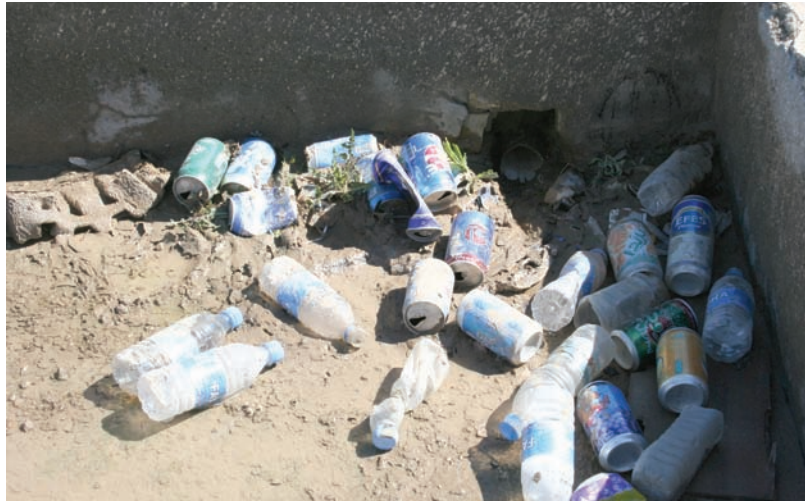
Roof drain blocked by debris.
