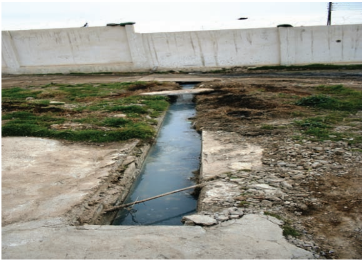
Open sewer culvert through station grounds still present, therefore not complying with the contract requirements.
