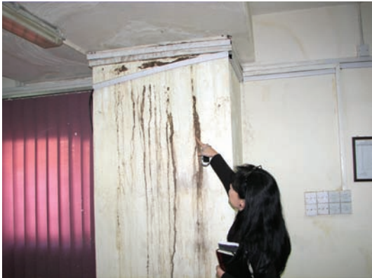
Water damage in ground-floor Operations Room.
