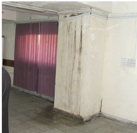
Water damage within the ground-floor Operations Room from SIGIR's first site visit in January 2007.
