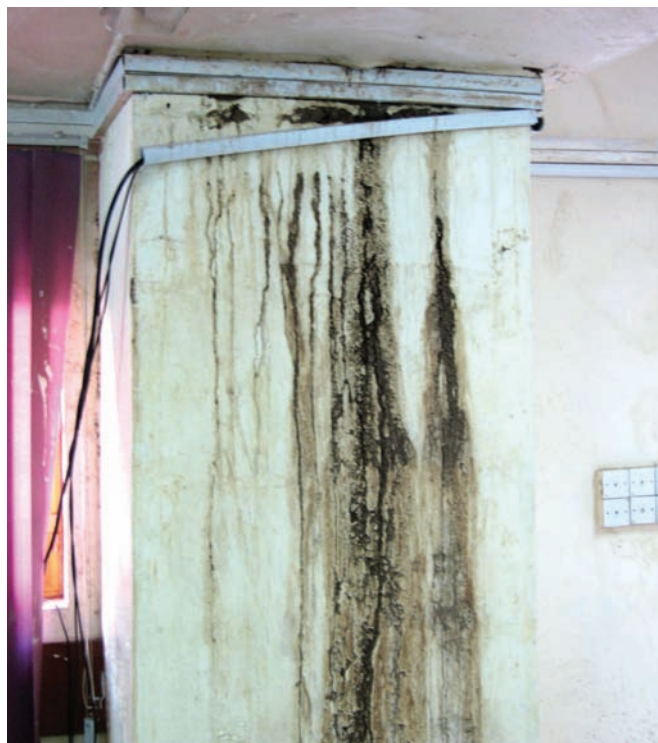
Significant increase in water damage between January and March 2007.
