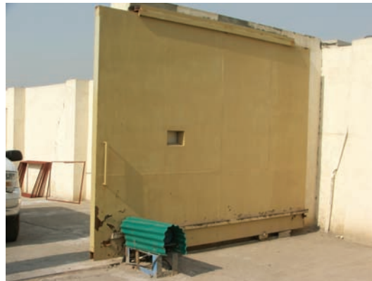
Right side of sally port gate, showing installed motor and two wheels to move gate. Significant amount of rust was noted.
