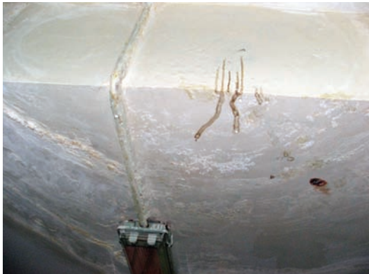
Close-up view of water damage on ceiling.
