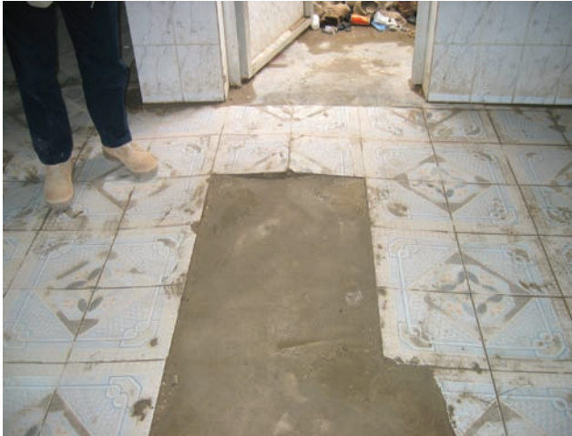
Buckled bathroom floors at inspection.
