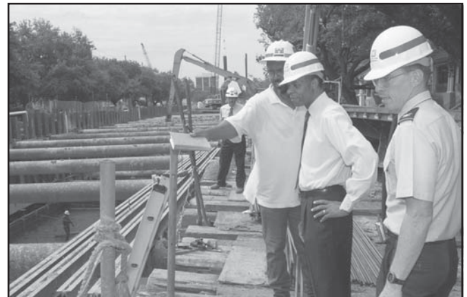
Construction inspector Leroy Smith (L) updates Congressman William J. Jefferson (C) and new U.S. Army Corps of Engineers District Engineer Colonel Peter J. Rowan (R) on progress of the Southeast Louisiana (SELA) drainage project near Napoleon and Claiborne Avenues. Budget constraints threatened continued progress on SELA drainage projects at the end of FY02. Additional funds were secured to continue the projects and to prevent potential public safety problems, while Congress approved an additional $32 million for the SELA drainage projects next year.
