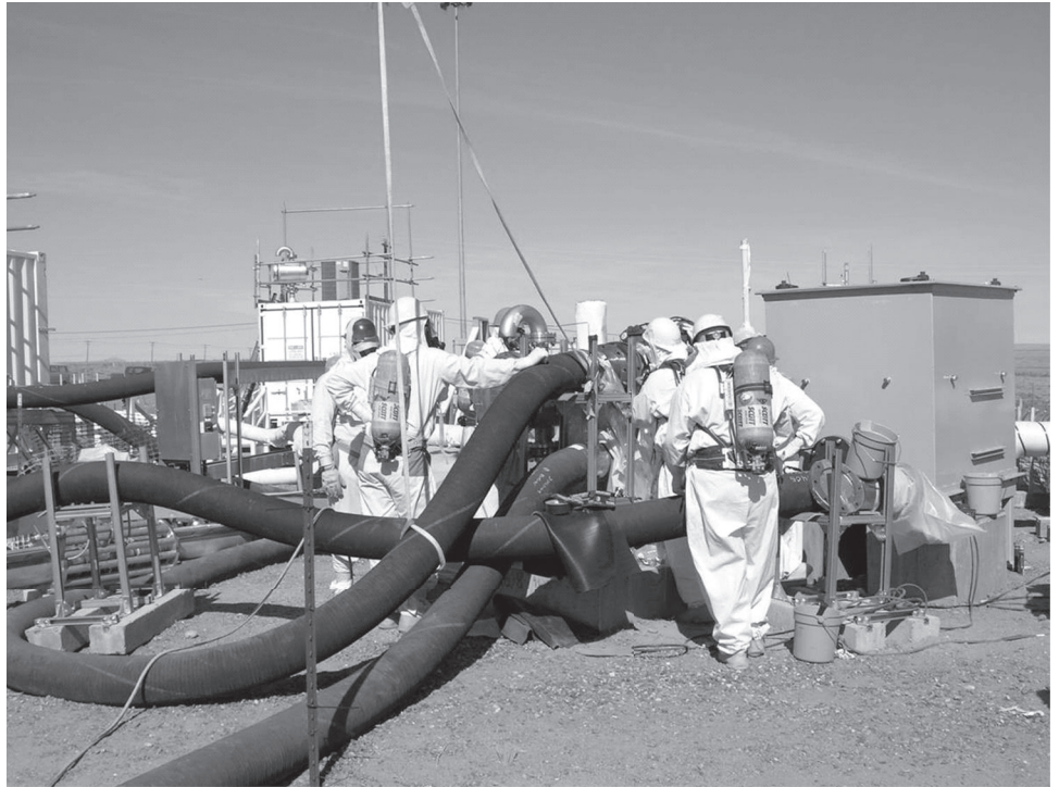
Figure 2: Workers Changing Out Equipment at the Tank Farms at the Hanford Site, a Hazard Category 2 Facility
