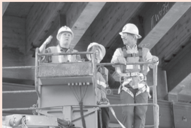
ODOT workers brief Rep. DeFazio on a failing I-5 bridge, part of a $4.7 billion bridge problem.
