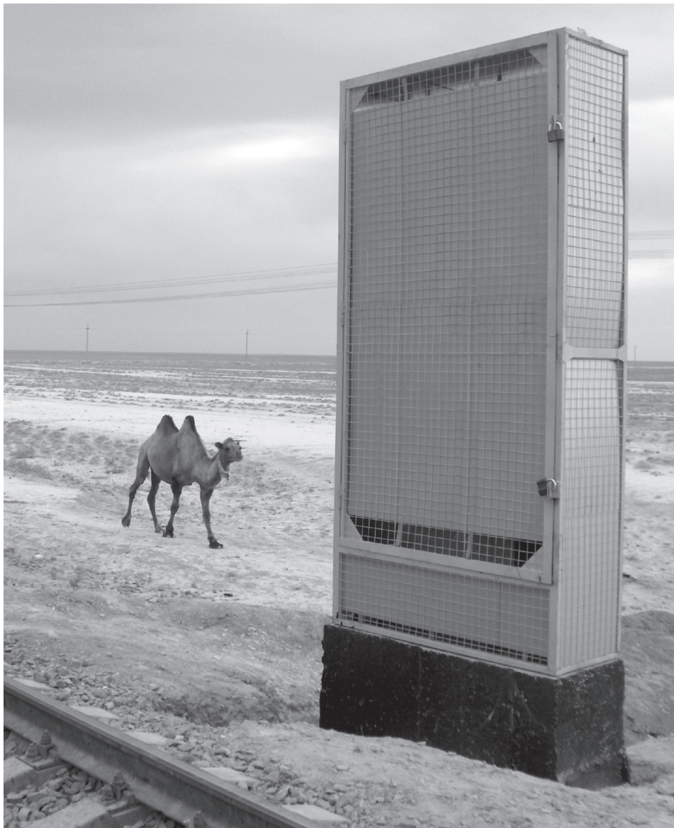
Figure 4: Rail Portal Monitor in Western Uzbekistan with Antitampering Protection
