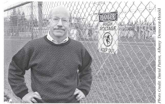
Rep. Defazio in front of a Bonneville Power Administration substation in Albany. He was one of 60 in Congress to oppose energy deregulation.
