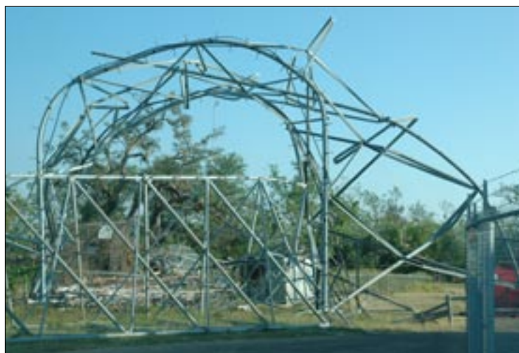
A downed communications tower, Plaquemines Parish, LA.
