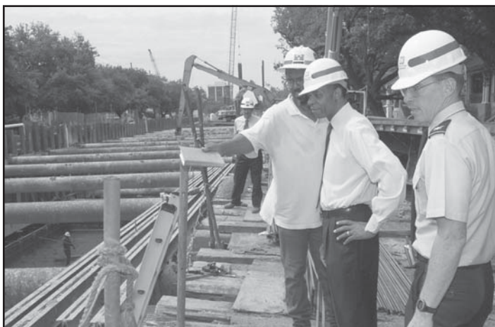
Congressman Jefferson inspects work on the Napoleon Avenue SELA flood control project with Construction Inspector Leroy Smith (L) and Colonel Peter J. Rowan (R) from the U.S. Army Corps of Engineers.
