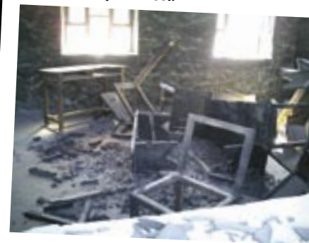
Taliban destroyed school.
